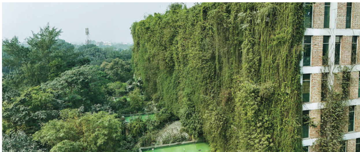
Photo 31: View of the Southern façade of the Karupannya factory building covered in dense vegetation
