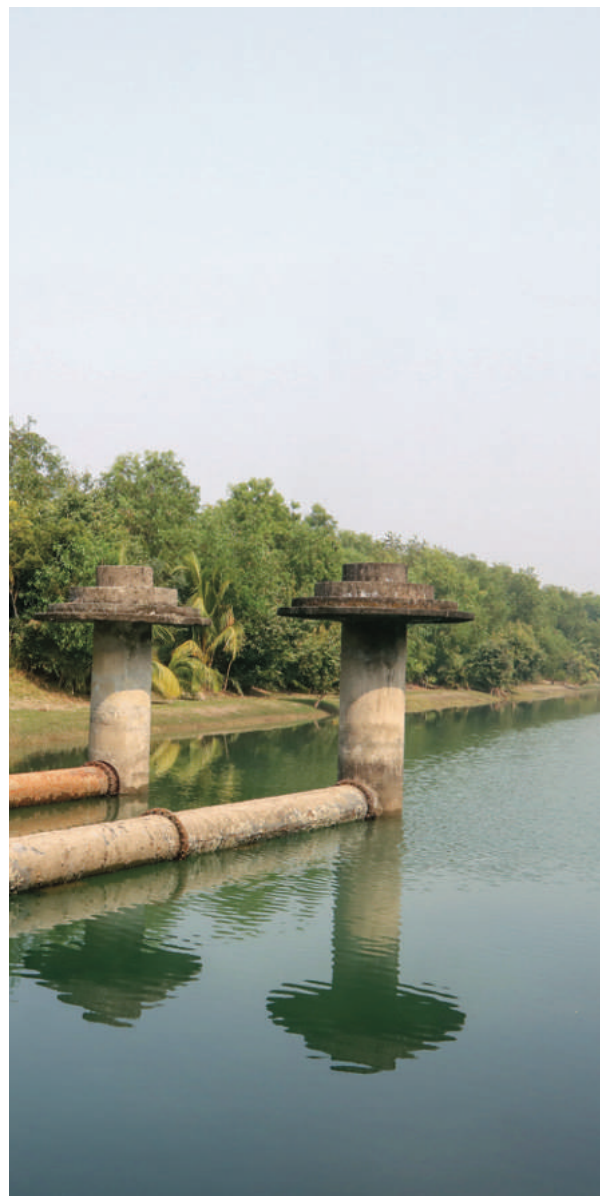
Photo 47: The edges of the ponds are covered in vegetation
