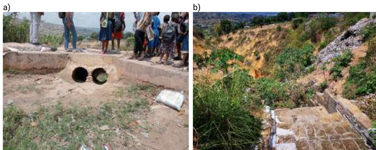
Figure 10. a) Circular channel for water evacuation; and b) sandbags in cascade created by the community.
