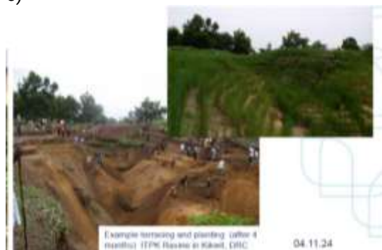
Figure 15. a) Terracing techniques in very steep slopes (greater than 50%) using seeding on the upper part and with riprap or vegetated gabions at the toe of the slope (left), or seeding of the entire sloping surface, reinforced by geotextiles or synthetic geogrids (right); 41 b) Vetiver plantation within sandbags in Brazzaville; 42 and c) Terracing example in steeper slopes in Kikwit, DRC. 43
