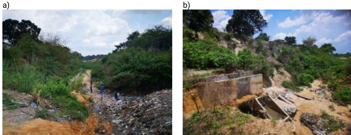
Figure 8.a) Western gully with vegetation along slopes; b) Incomplete dissipation tank in Ngambio.
