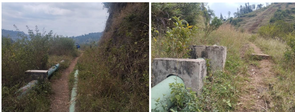
Figure 12: Water Supply HDPE pipes anchored by reinforced concrete anchors along the foot of the slopes to deter impacts of landslides and rock fall at Irate Intake. Second phot also show evidence of poor slope clearance and cultivation
