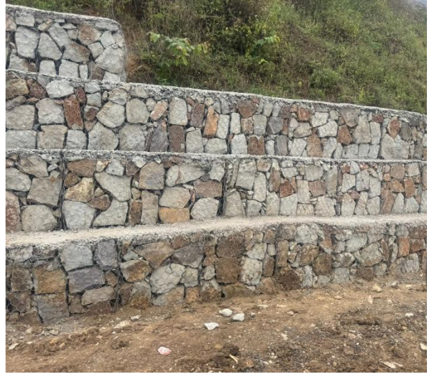
Figure 21: Slope Stabilization Gabions along a slope in Murang'a
