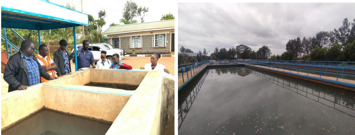
Figure 19: Sedimentation and Dosing Chambers at the treatment plant
