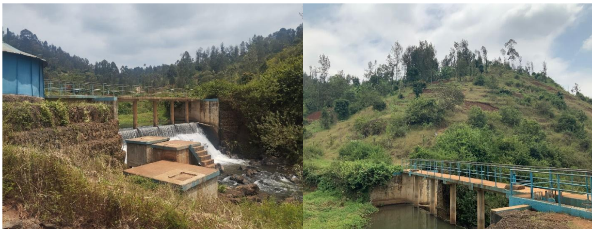
Figure 10: Irate Intake on River Irate in Gachocho area.
