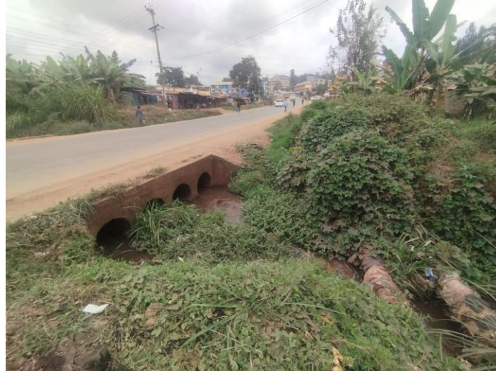
Figure 18: Sewer pipes crossing River Gathamba near Muwasco Offices.
