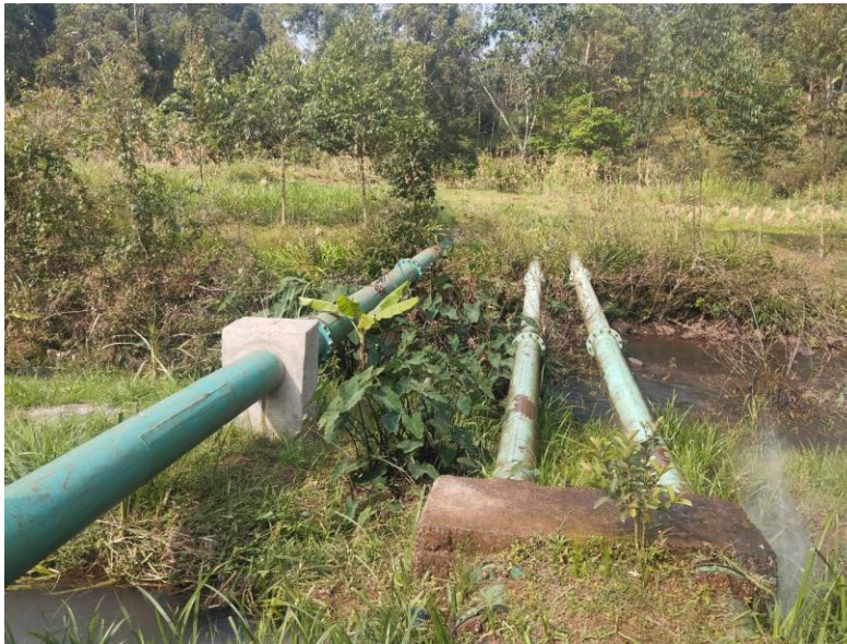
Figure 15: Relocated pipes running along River South Mathioya valley in Kiarathe with river crossing fitted with GI pipes from the joint chambers and firmly anchored by concrete reinforced anchors.
