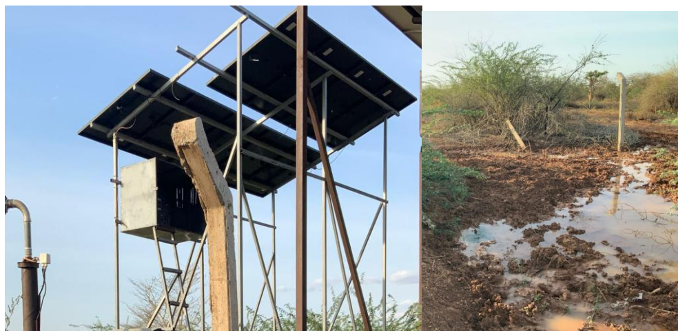
Figure 21: Stolen Solar Panel and Broken Water Pipe in Madogo.
