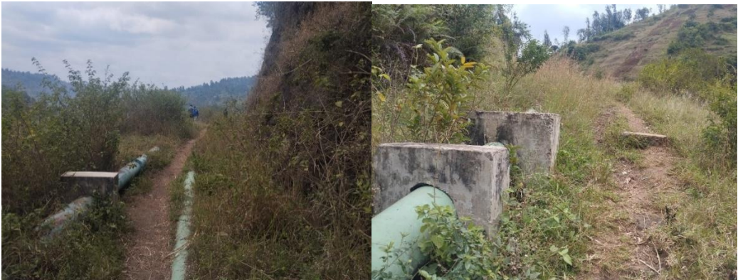
Figure 50: Water Supply HDPE pipes anchored by reinforced concrete anchors along the foot of the slopes to deter impacts of landslides and rock fall at Irate Intake. Second photo also shows evidence of poor slope clearance and cultivation.
