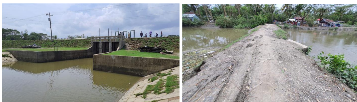
Figure 6.2: Three-vent sluice gate over the Khaprabhanga River (left), and the Khajuria Khal and Alipur Khal have been detached due to the construction of a road with a narrow opening (right)
