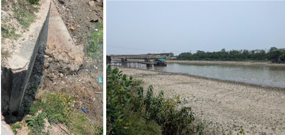
Figure 4.4: Failure of sluice gate at polder 31 (left); Water treatment plant of Chalna Pourashava at Vadra River (right)
