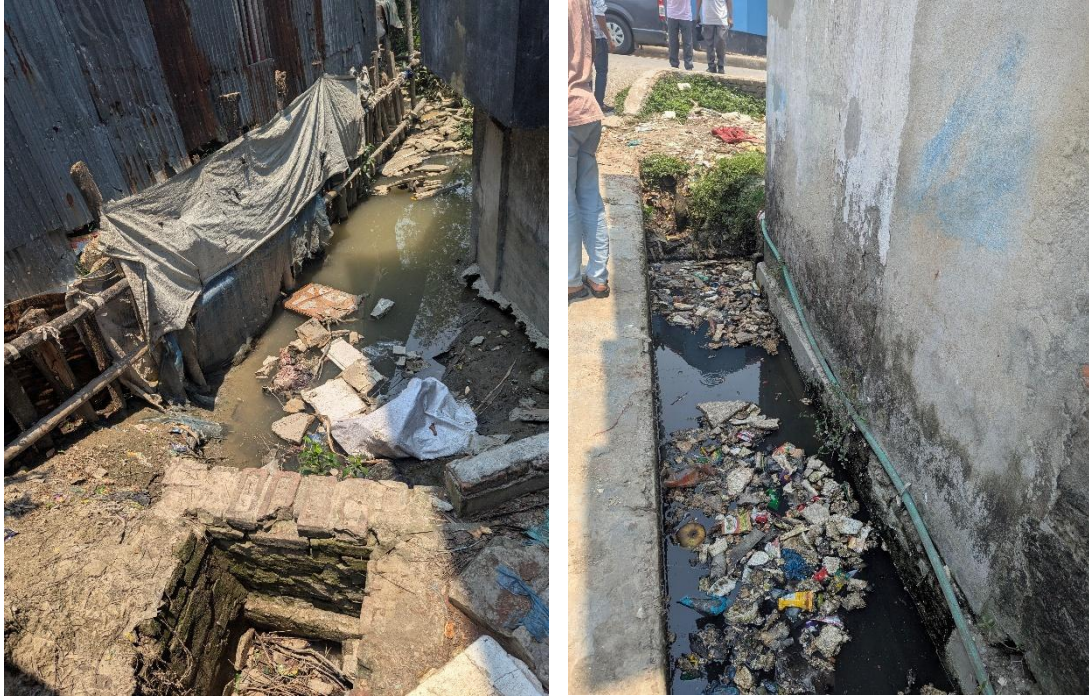
Figure 3.3: Dead sluice gate (left) and clogging due to the dead sluice gate (right)
