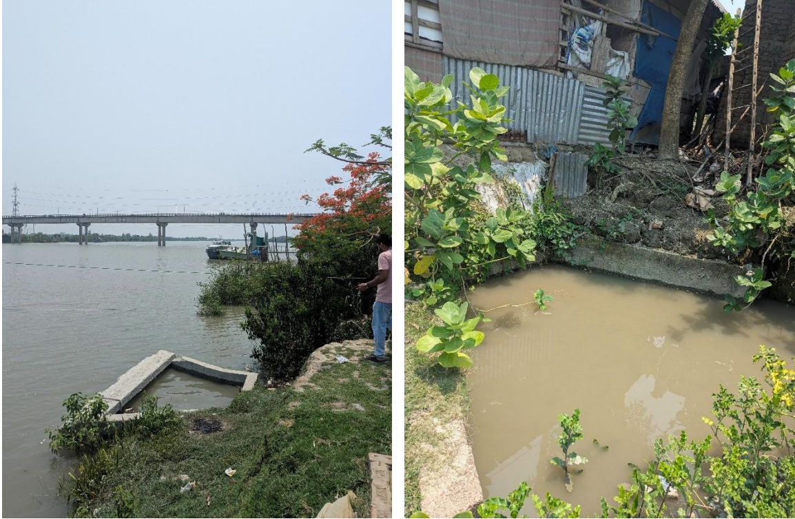
Figure 3.4: Under-capacity functional sluice gate
