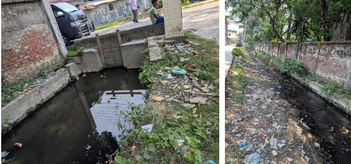
Figure 3.2: ill-maintained drain with an improper sluice gate (left) and an open drainage system (right)
